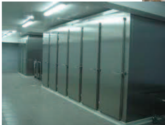
Refrigerators in a mortuary
