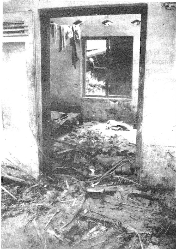
Plate 4: (A) Damaged rooms in one of the houses shown in Plate 3 (B). (B) rock and other debris of the same landslide of Plate 3.
