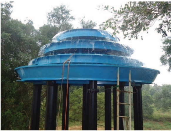
Figure 5 Cascade aerator made by NWSDB
