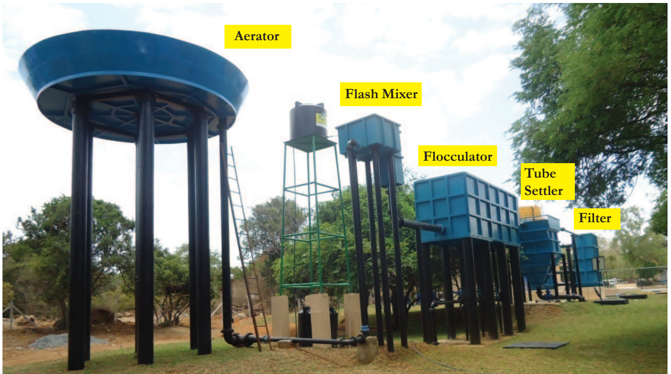
Figure 16 Conventional water treatment plant at Thanthirimaley (A joint effort by the Research & Development Unit, the central workshop and the Anuradhapura regional Office of the NWSDB)
