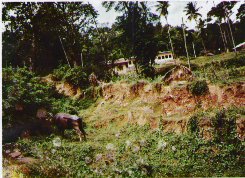
Fig. 3 Pooliyadda Creeping Slope Failure with Damaged Buildings of Weldambala School in the background.
