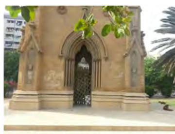
Figure 14: Broken door, wall chalking & posters
