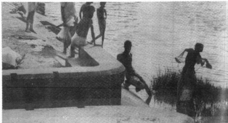
An anicut in the downstream areas for regulation of water flows for irrigation
