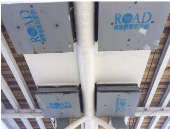
Figure 4: TMD under the girder
