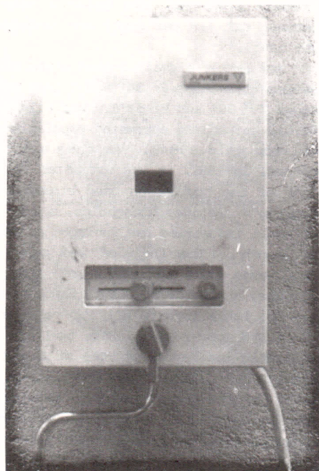
Hot water Unit operated with Biogas at Wewandon Estate Nuwara-eliya.
