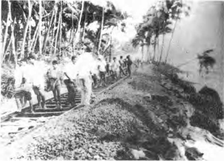
Figure 4.3: Coastal erosion along the south-west coast showing damage to the main railway line to Galle (Picture by ANCL).
