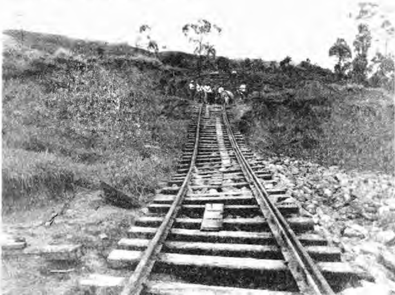
Figure 5.1: The recurrent landslide at Watawala showing the serious damage to the upcountry railway line.
