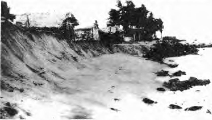
Figure 4.2: Coastal erosion along the south-west coast showing damage to houses and to land (Picture by ANCL).
