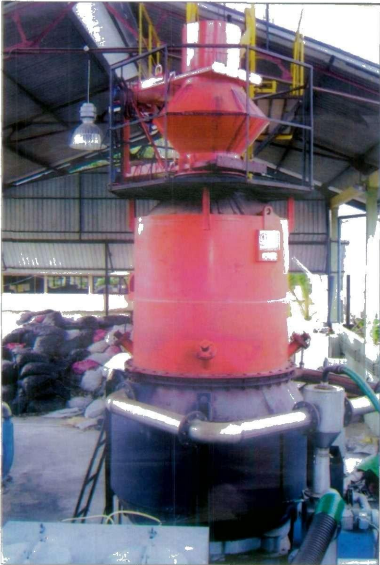
Dendro power plant
