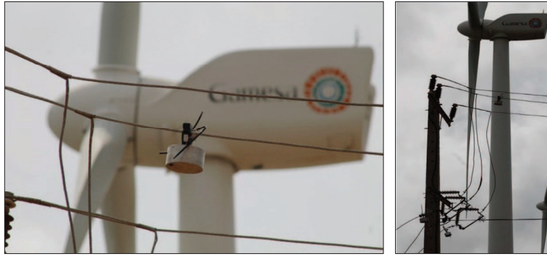
Figure 8: Devices mounted on a wind turbine collector conductor
