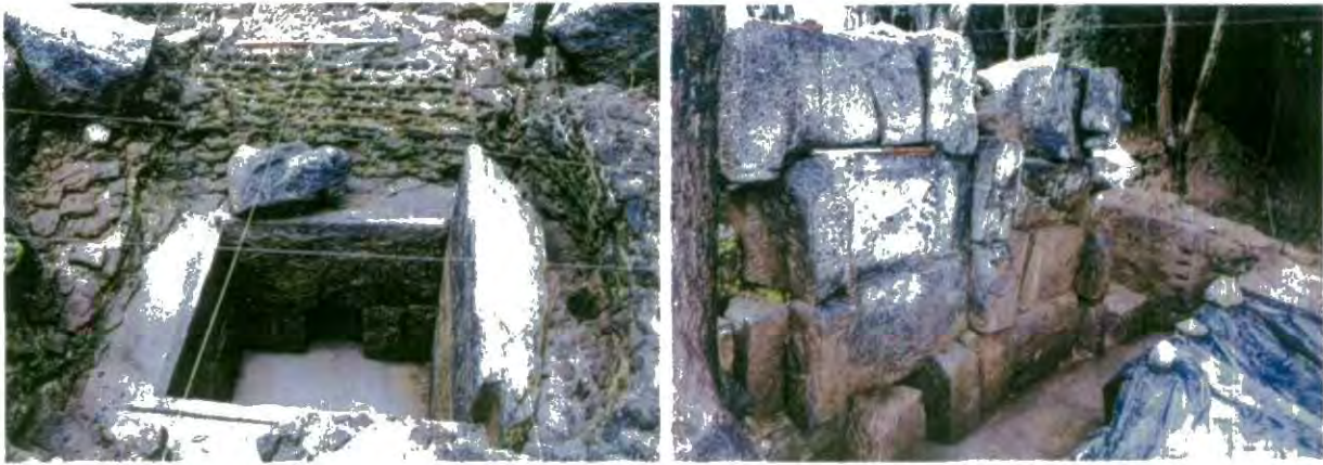
Plate 8: Bisokotuva at the ancient Buvava near Parakrama Samudra and inlet Culvert of the Bisokotuva
