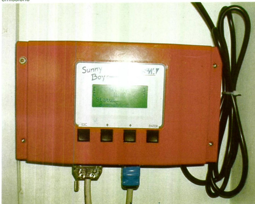
Inverters convert the DC current generated by the solar panels into AC for supply to the national grid.
