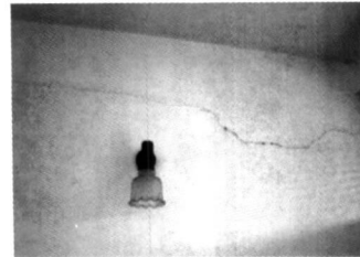
Figure 6: Horizontal cracking under beams
